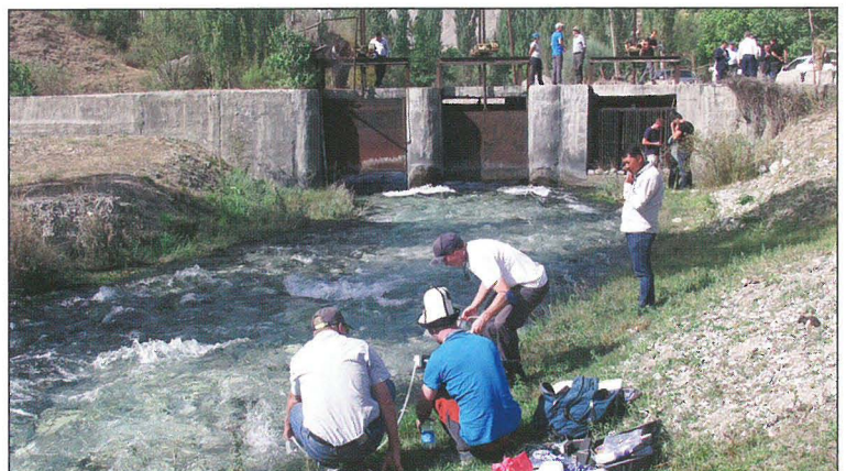
Existing intake structure for the planned Shakimardan SHP on Koxsu river in Uzbekistan
